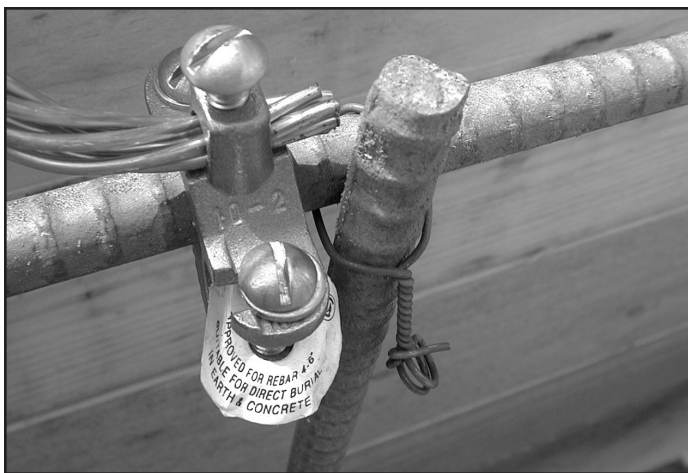
Figure 4 — Ground Clamp inside Foundation
